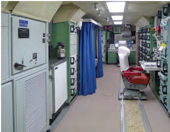
The interior of the D-1 LCC acoustic enclosure. Note how much smaller it is than that at O-0.
